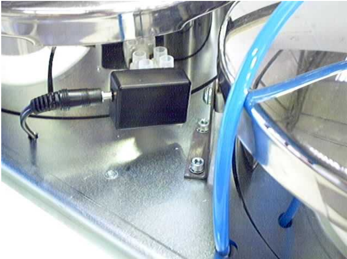
Figure 2. Jack Plug incorrectly fitted to Digitizer
